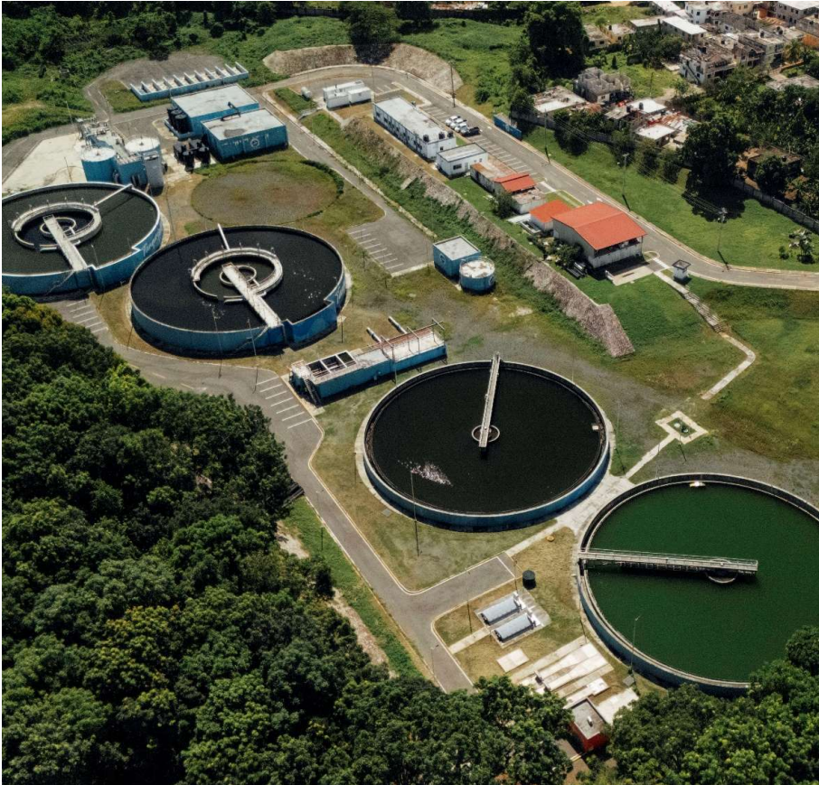
Wastewater treatment plant in Dominican Republic, part of a sanitation and sewerage infrastructure improvement project financed by AFD.
